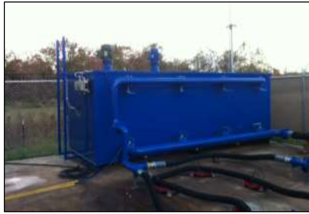
Figure 4: Mud Tank (Four 1000 gal. segments)
